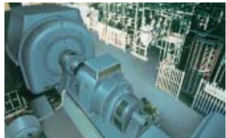
Short-circuit test generator No.1
